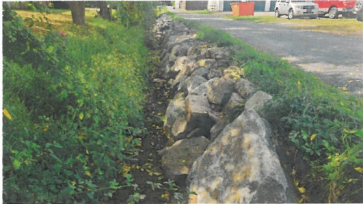
Rip Rap was added to the bank of the Loyalt- ton Run to stop erosion into the roadway.
