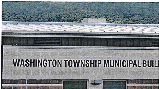
New Roof was installed on the Office part of the Township Building this Spring
