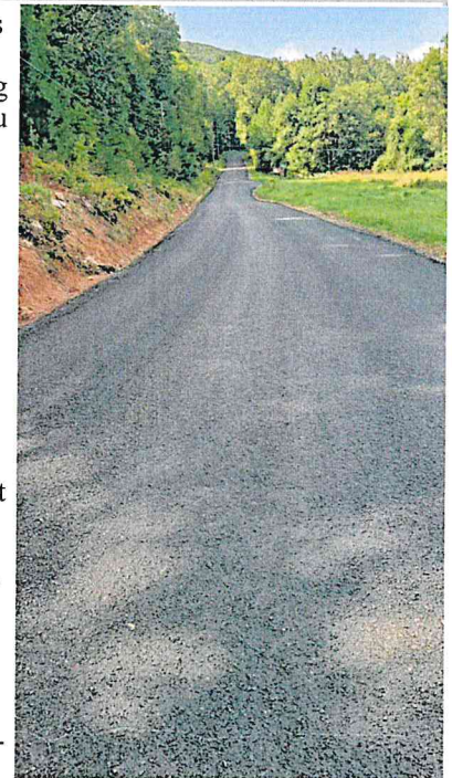
Mohr Road, the berm was widened and the roadway was Seal Coated and Fog Sealed.
