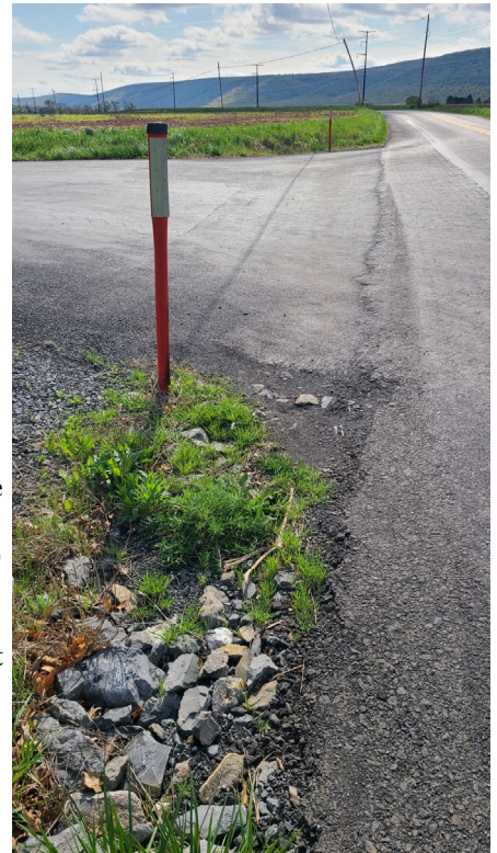
Drainage Project on Henninger Road has eliminated the water ponding and Ice build up during winter
